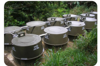
Waste Treatment System
